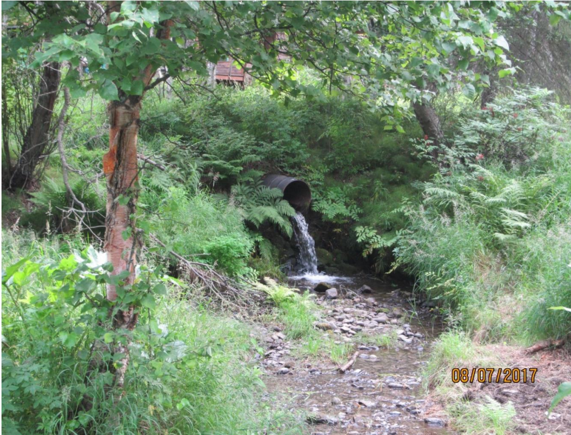
Fig. 44 Perched culvert on S. Fork Little Campbell Creek just east of the Alaska Zoo’s boundary (2017)
