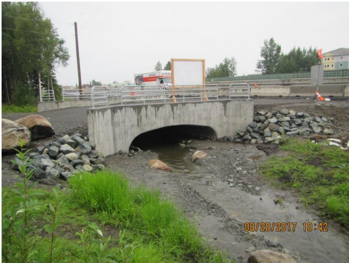
Fig. 40 View of the new driveway and large culvert at 70 th and Homer over N. Fork Little Campbell Creek looking north (2017)
