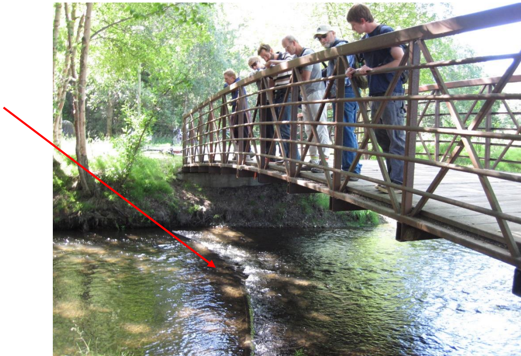
Fig. 11 Exposed utility line in Chester Creek at Karluk (CW-11) during field survey in 2012
