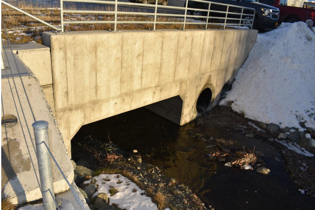
Fig. 43 S. Fork Little Campbell Creek, New Seward Highway culvert replacement at Brayton looking north as the culvert makes a turn to the west under the driveway over the creek (2019)
