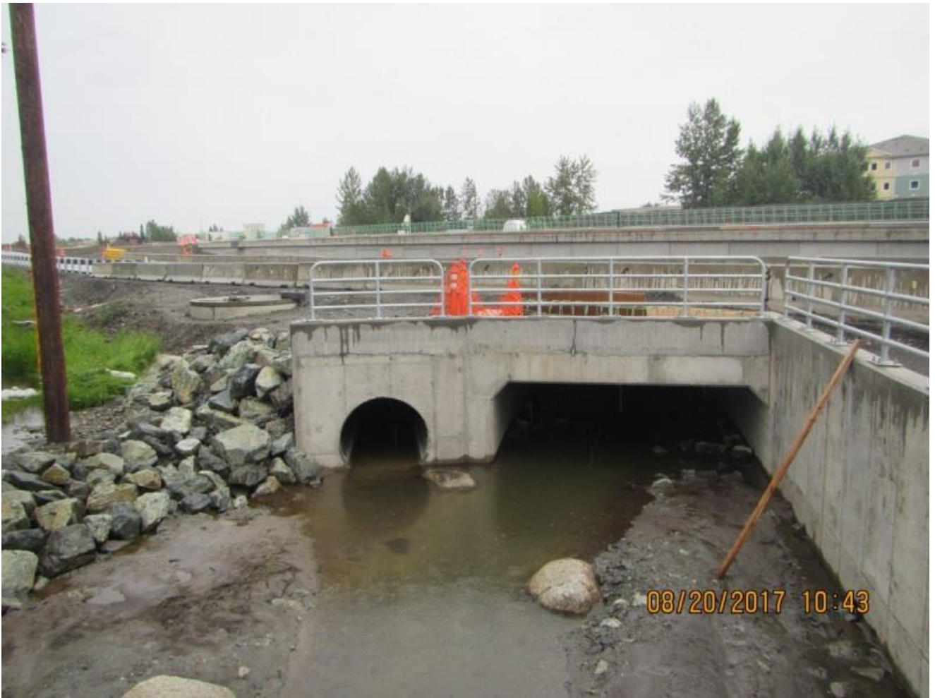
Fig. 38 New box culverts at N. Fork Little Campbell Creek outflow looking east under the New Seward at 70 th and Homer (2017)
