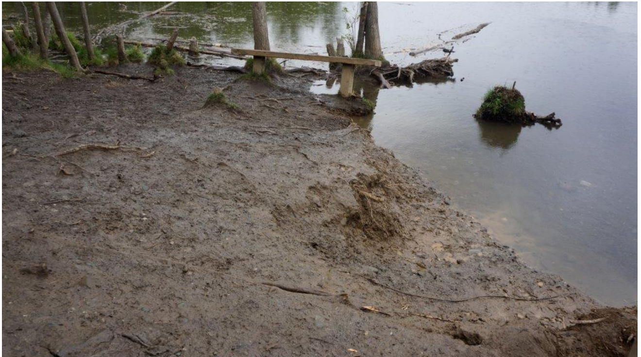
Fig. 18 Bank erosion in 2016 near foot bridge at S. Fork Chester Creek inflow to University Lake, CSF-4
