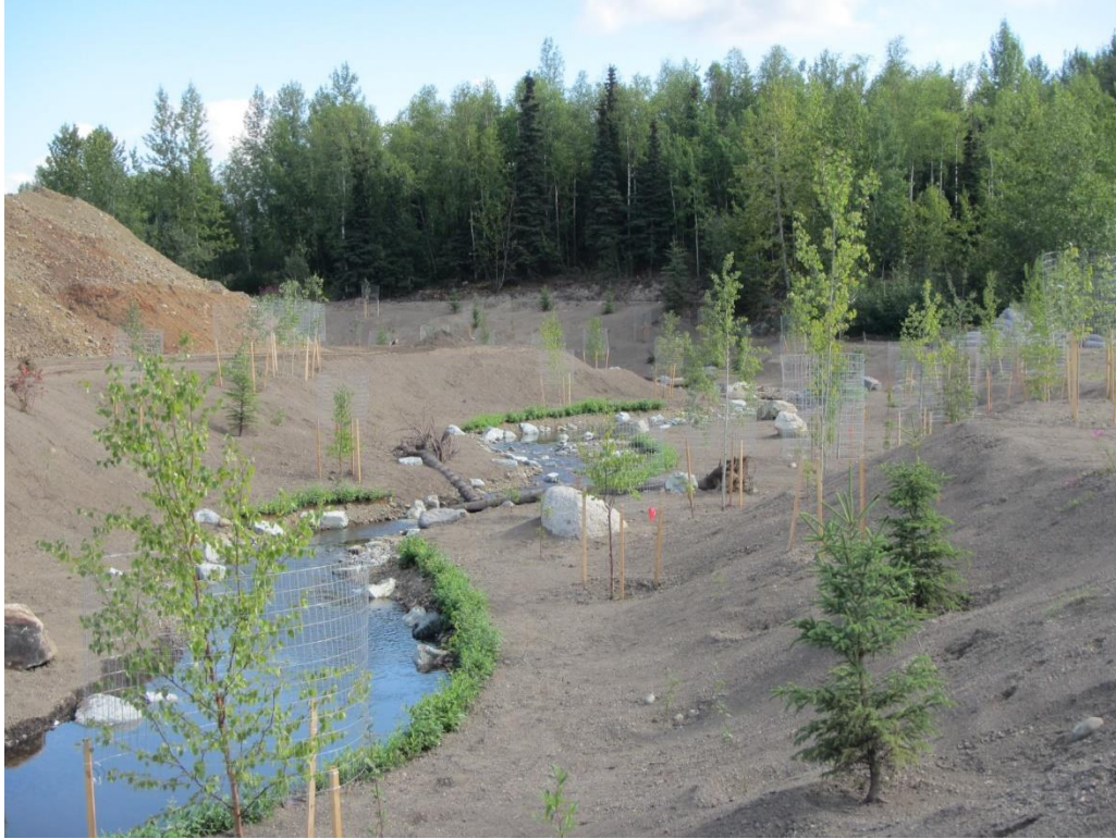
Fig. 32 Looking east from Muldoon at the former Greenhouse property after creek alignment (August 2015)
