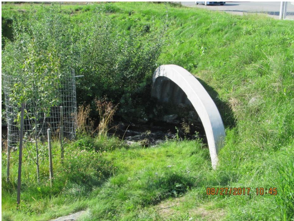
Fig. 29 New culvert on realigned S. Fork Chester going west under Muldoon about 550' from old culvert (2017)
