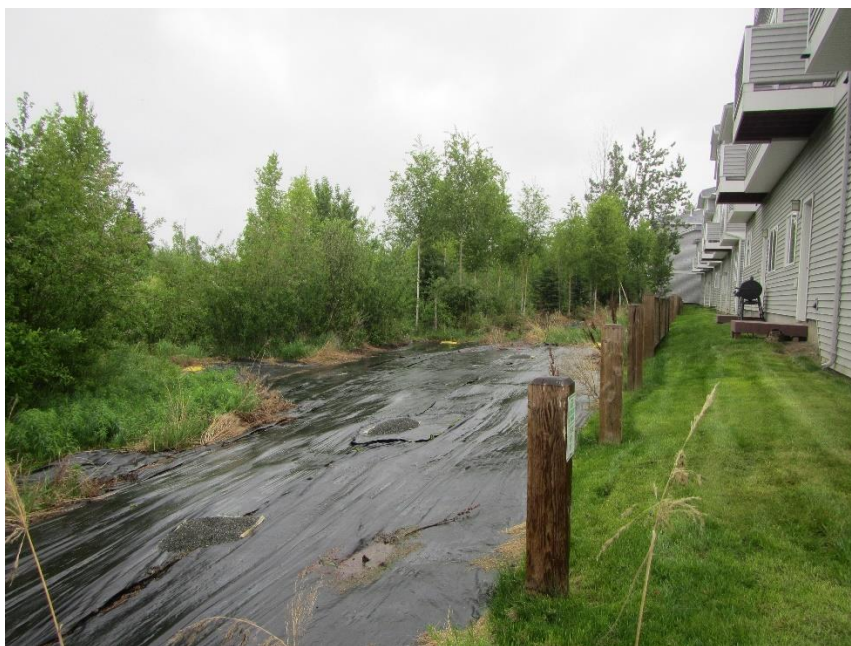
Fig. 20 Area still covered with tarping near S. Fork Chester Creek in June 2015
