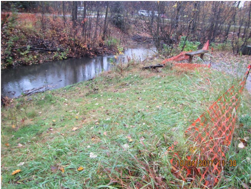
Fig. 14 North bank of S. Fork Chester Creek at University Lake outflow under Elmore in 2017 after 2014 bank restoration, CSF-4
