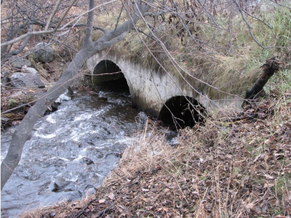
Fig. 28 Old culverts on S. Fork Chester original channel going west under Muldoon (2009)
